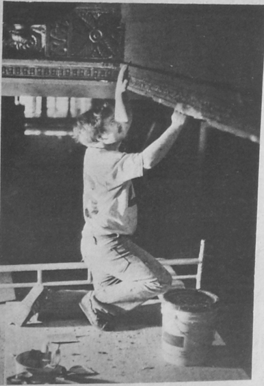
Glenn Hinchey, an employee of Crown Restoration, removes old paint from a wall surface.
